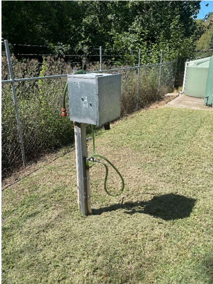
Services point at the steaming bays, includes 12V power and water.
