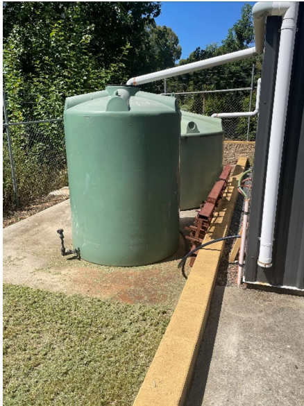
The water supply is via rainwater tanks. Water to the steaming bays is via a pump from the tanks to a tap at the services point.
