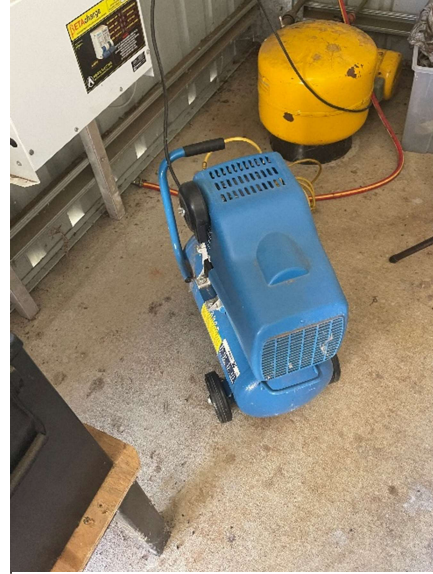
Compressed air is available.
